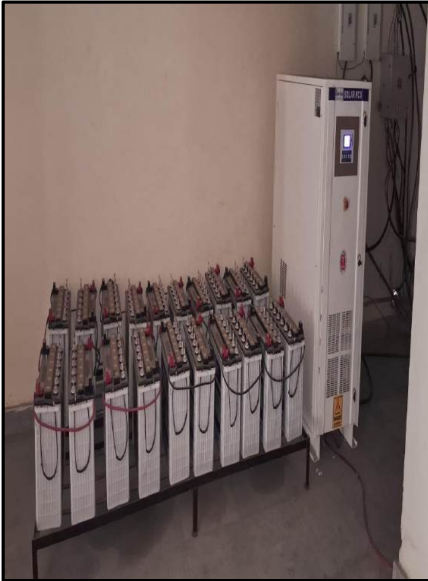
Solar Panel Batteries
