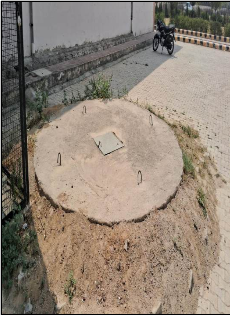
Rain Water Harvesting System
