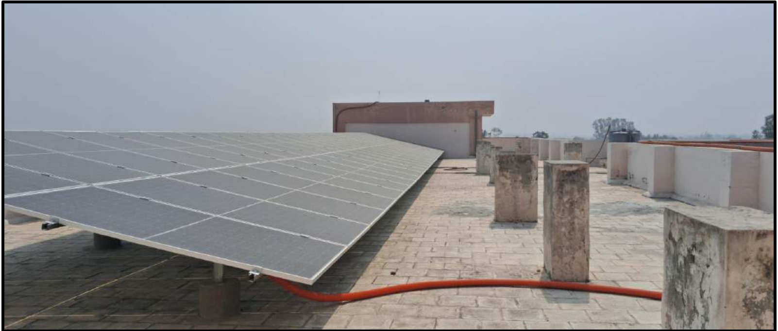
Solar Panel-28 KW
