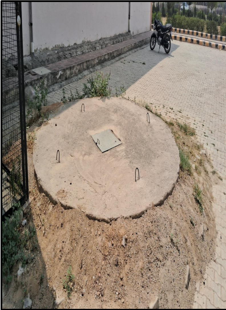
Rain Water Harvesting System
