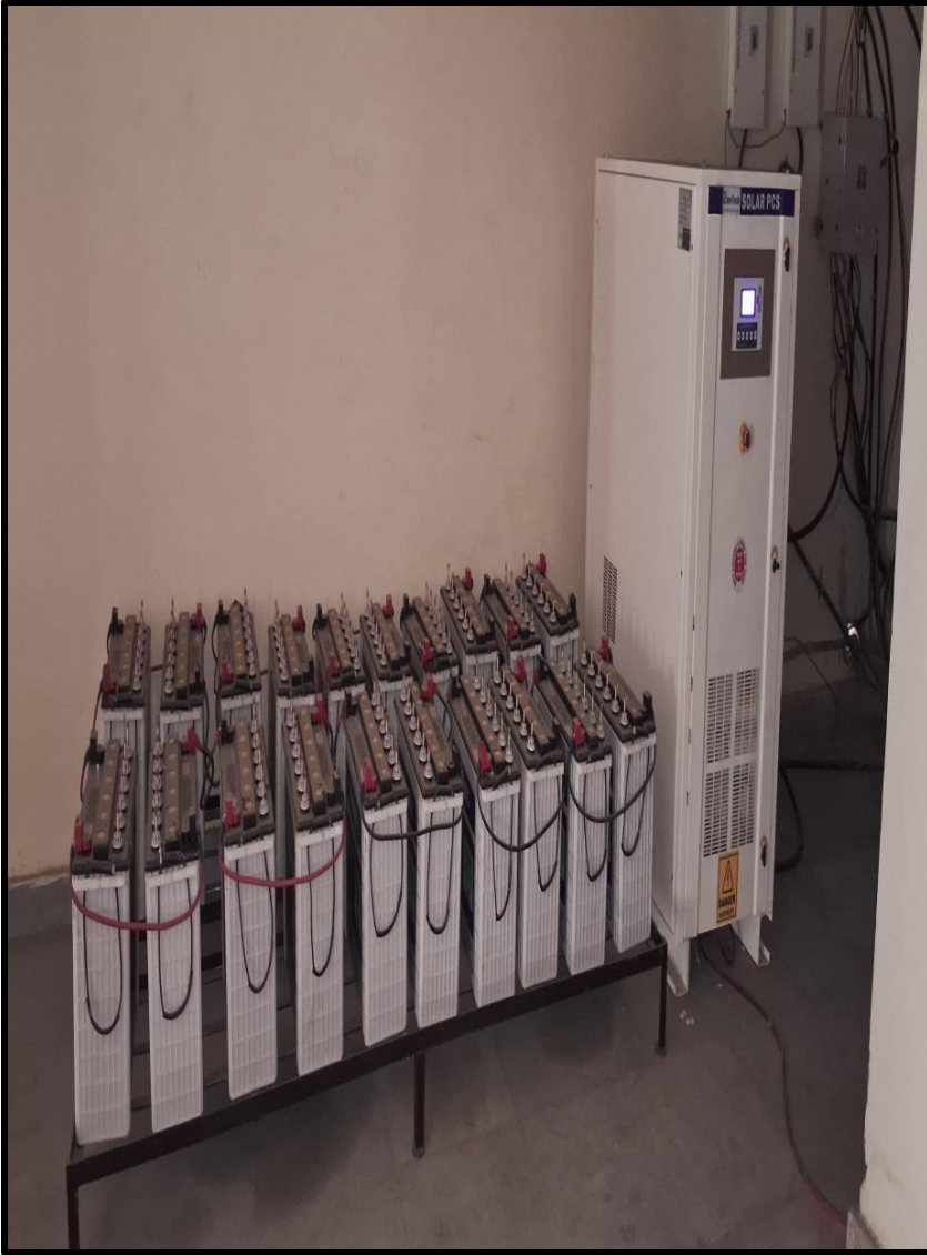
Solar Panel Batteries
