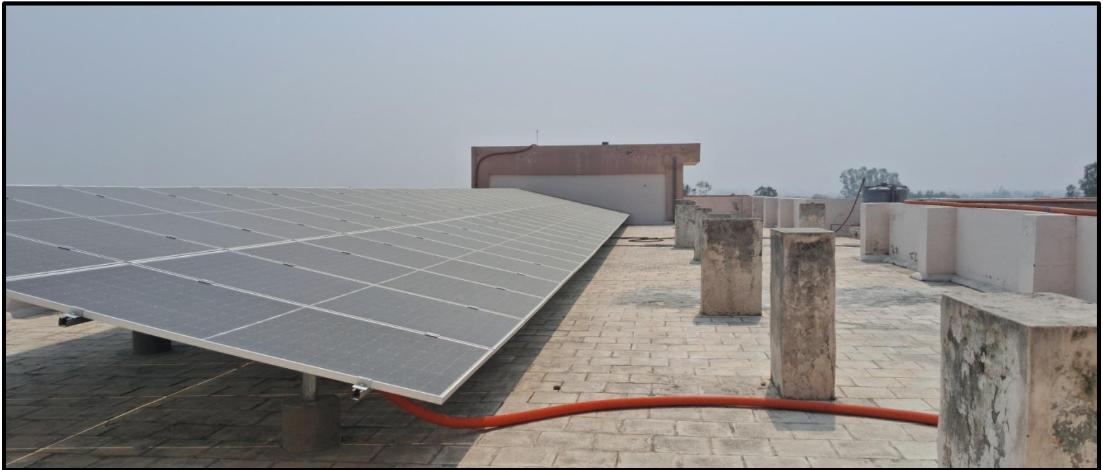
Solar Panel-28 KW
